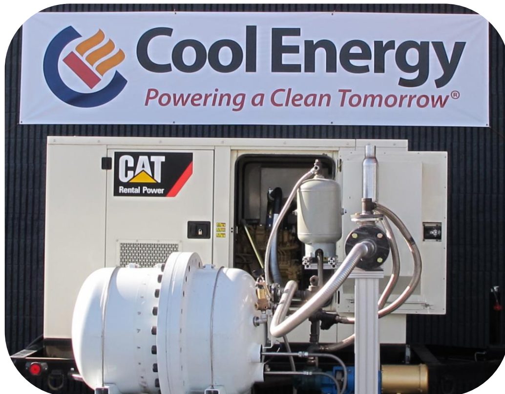
Fig 4) 3 kW e ThermoHeart® Engine boosting genset output by up to 7%.
